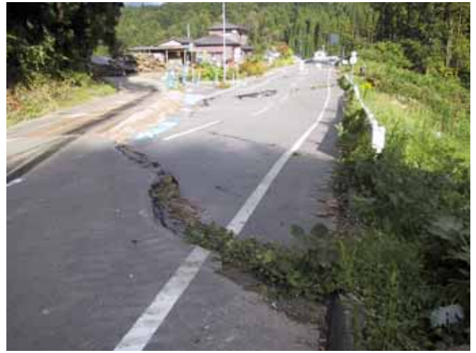
Figure 11. New cracks appeared on the road in May 2003.
