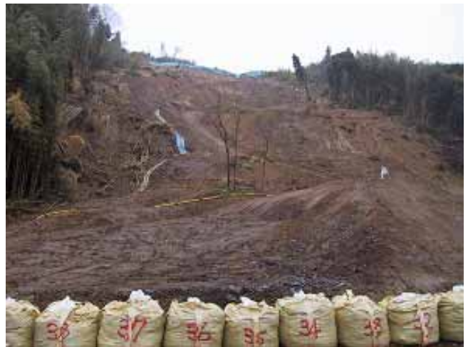
Figure 5. A closer look into Katanoo landslide as the effort to prevent further sliding was underway.
